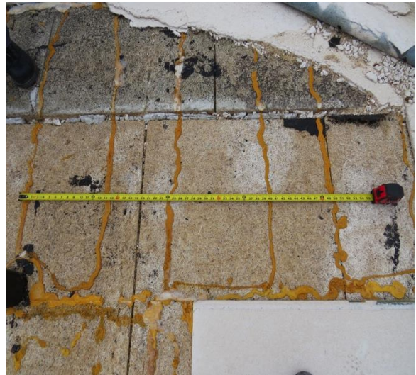
Foam Adhesive did not bond to gypsum board
