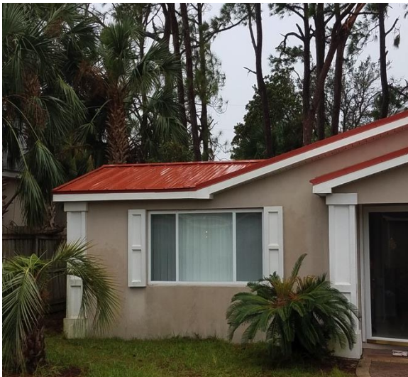
Damage from debris
