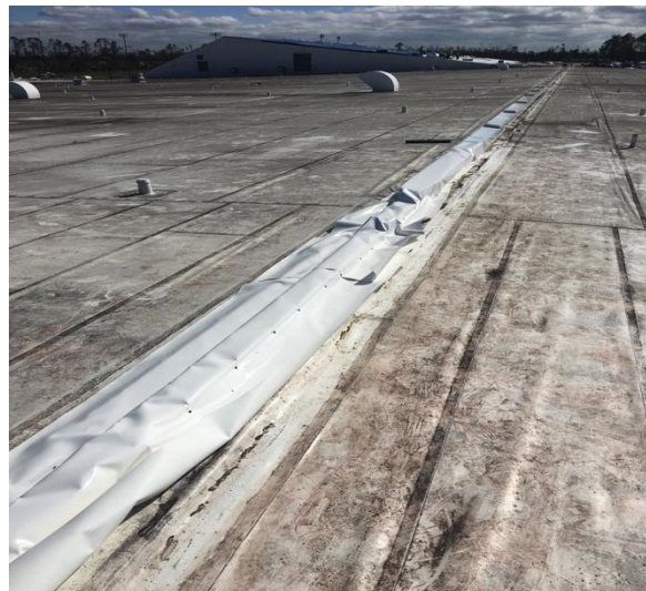
Dislodged divider coping
