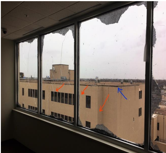
Glass broken by debris, sacrificial exterior layer shatters, interior layer may crack. Typical of all windows on the east side of this hospital tower.
