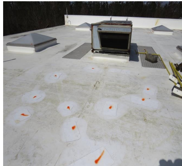
Other punctures from debris
