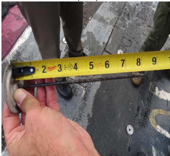
1.2.2 Fastener Some corrosion
