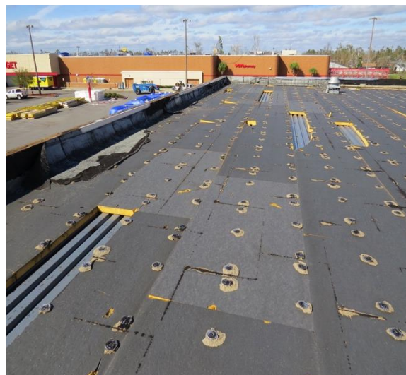
Insulation blown from deck
