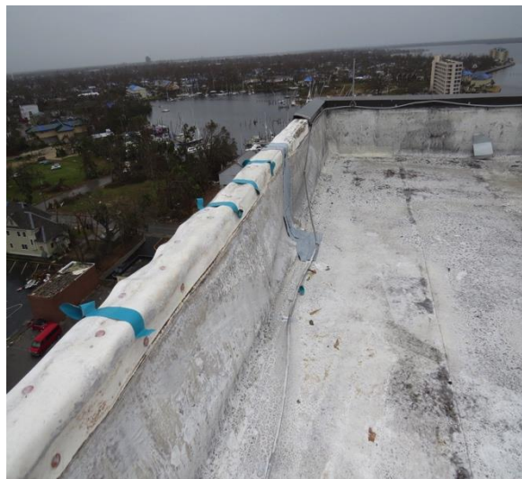
Missing Coping, bulge in parapet cladding
