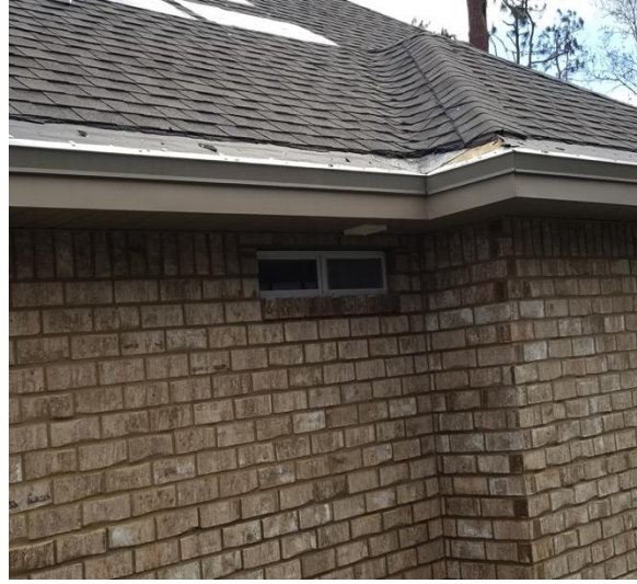
Starter row of shingles dislodged
