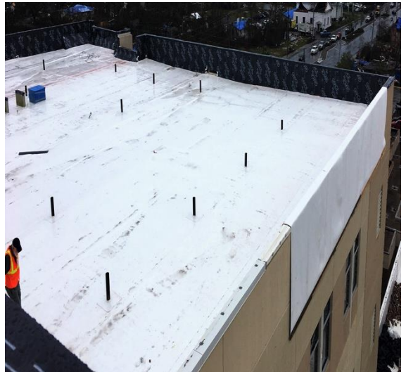
Large section of temporary parapet cover and roof membrane
