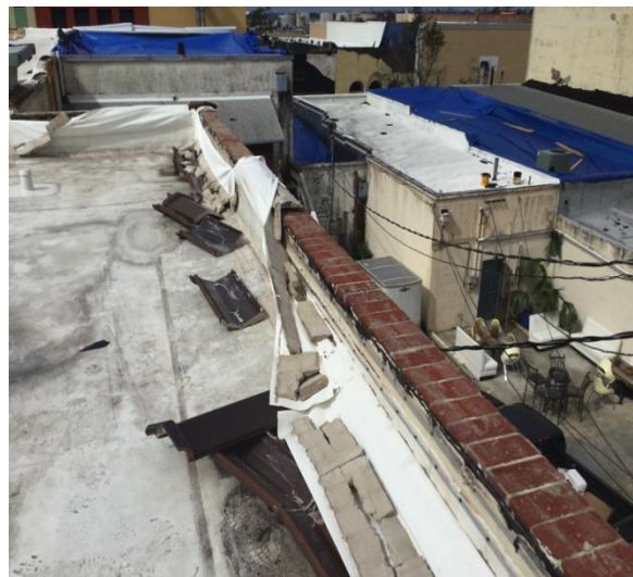
Membrane pulled paver from parapet
