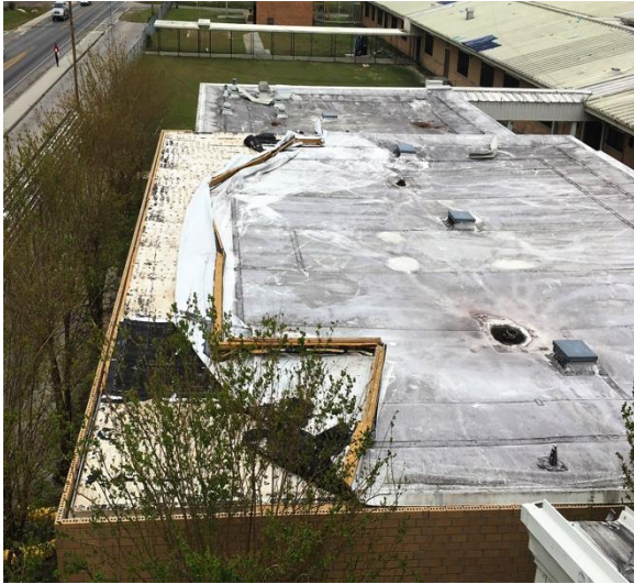
2.1.2 Overview entire edge dislodged
