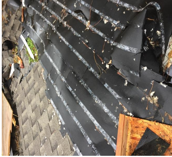
Nails pulled out.
