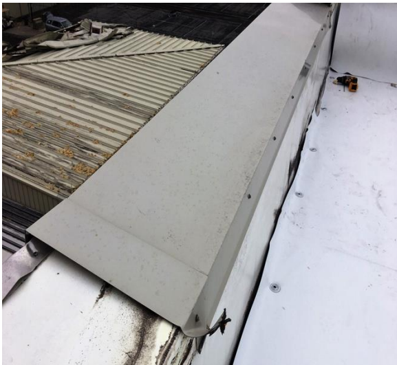
Dislodged coping on upper roof
