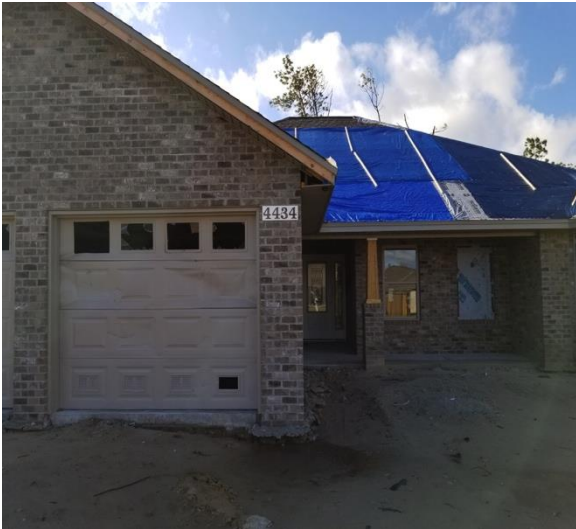
3.2.1 Front, Unusual area where shingles are dislodged
