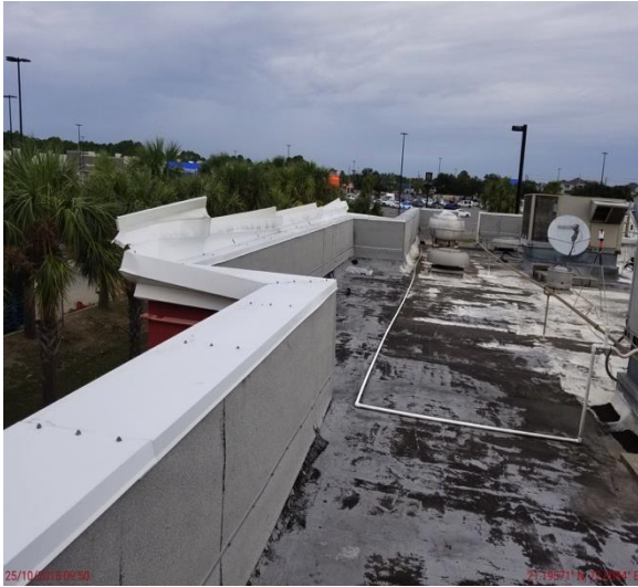
4.1.1 Overview with damaged coping
