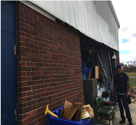
Collapsed Brick Wall
