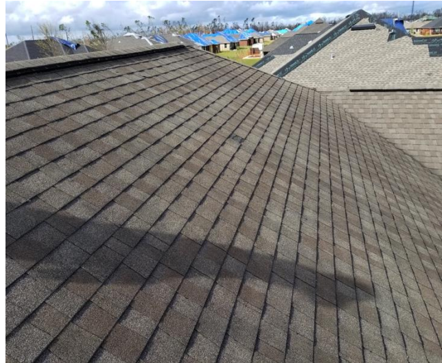
Overview: One broken shingle
