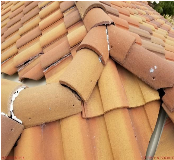
Ridge Tile – It is not clear how the tile were attached. Note: Nail holes and possible foam adhesive.
