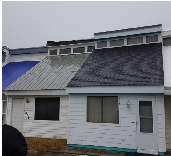
Only obvious damage is to soffit section on through fastened roof
