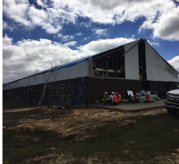
Collapsed wall and missing panels
