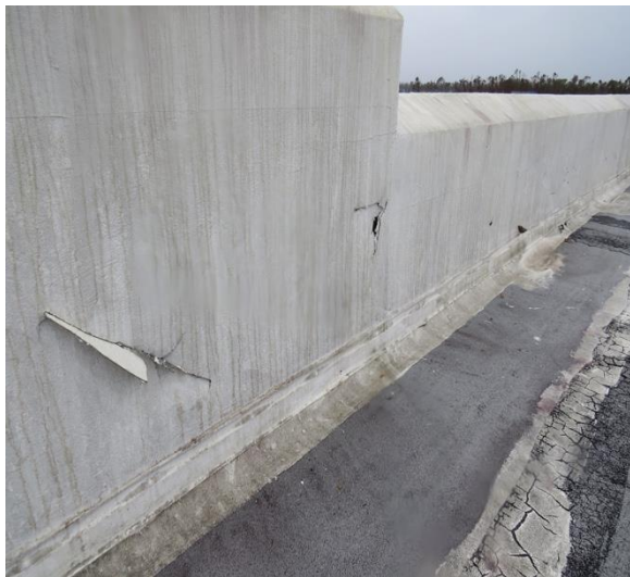
1.1.6 Puncture damage to parapet
