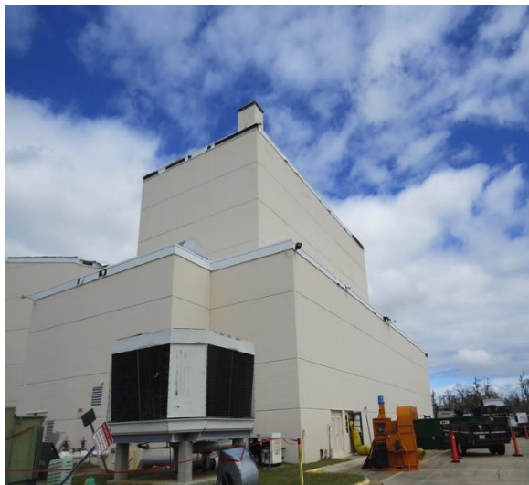
1.2.3 Outside overview showing missing coping
