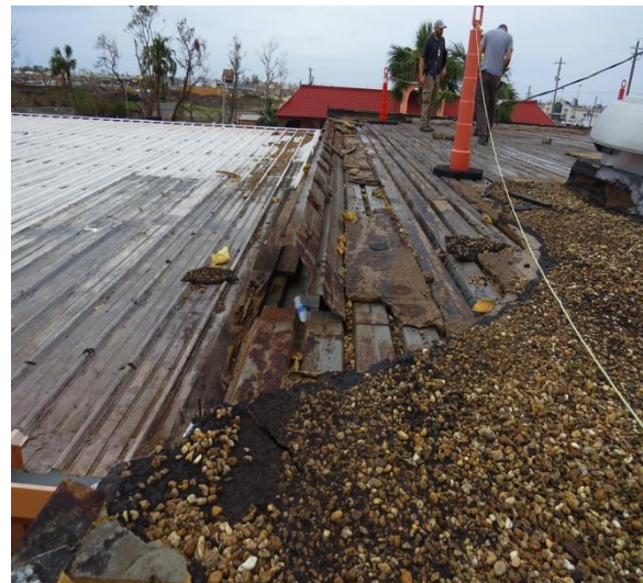
Overview of deteriorated system
