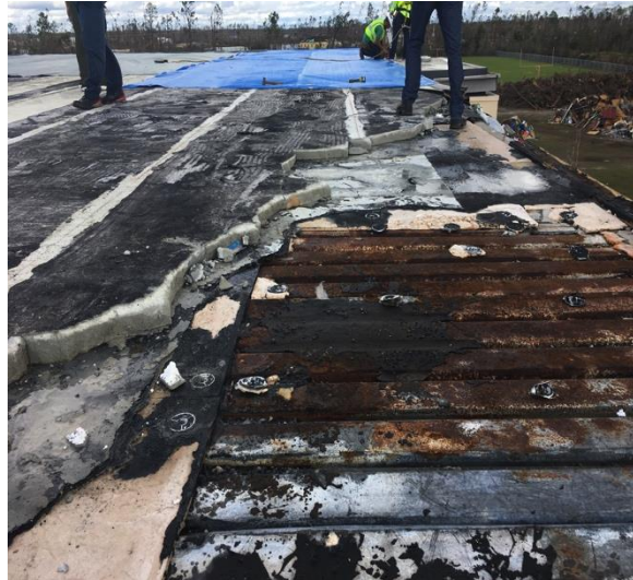
Rusted metal deck showing complete system
