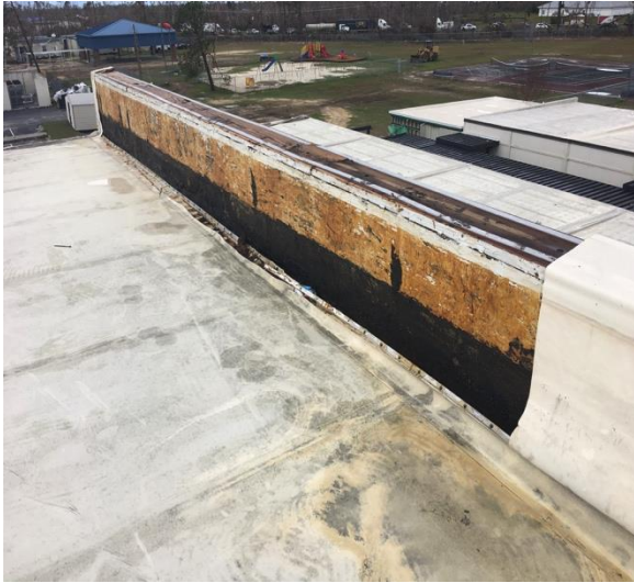
2.2.1 Coping and parapet wall flashing dislodged
