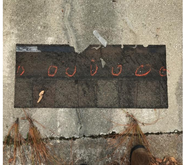
Shingles with 7 nails
