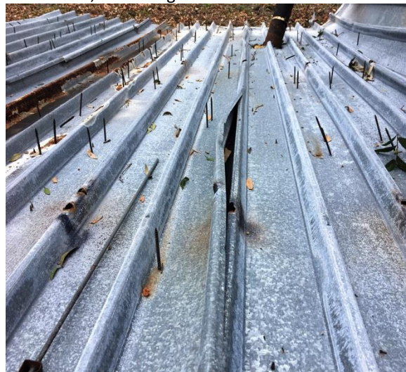
Deck welds did not resist the uplift.
