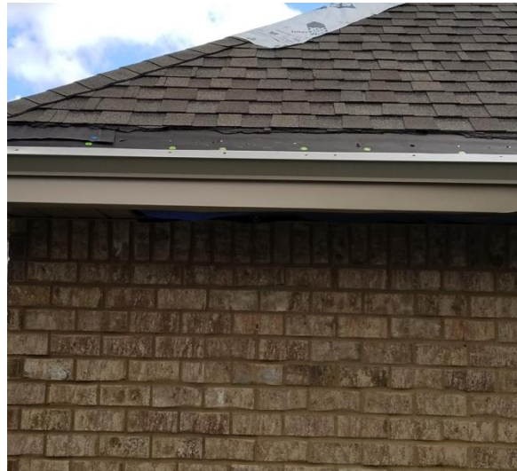
Starter Row missing
