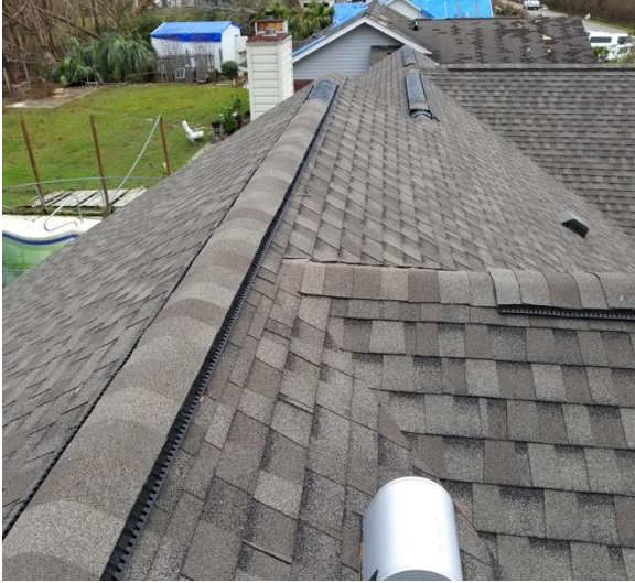
3.1.2 Overview indicating very limited damage
