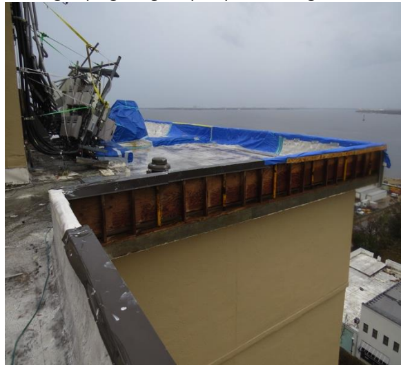
Missing Cladding over parapet
