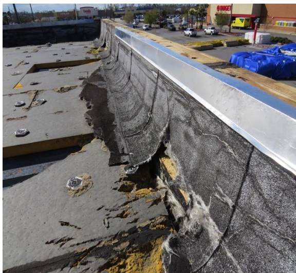
Membrane tore from wall
