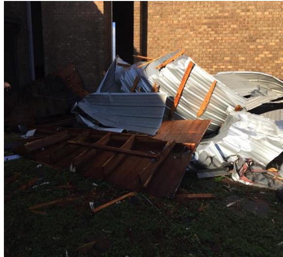
Debris showing deck and metal
