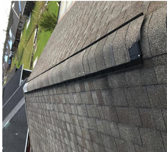
Broken ridge cap shingle
