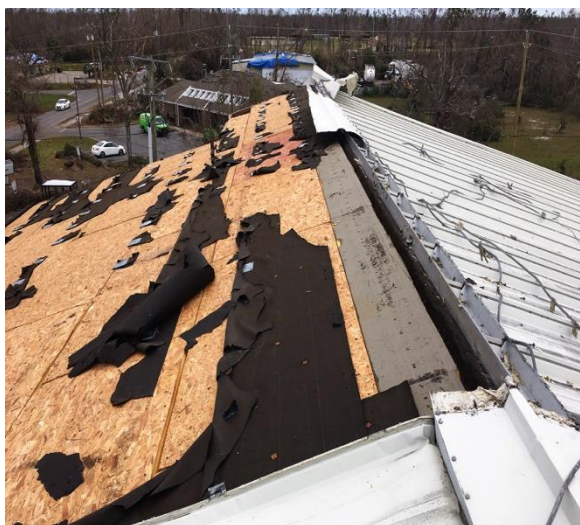
2.1.1 Overview of area of dislodgement
