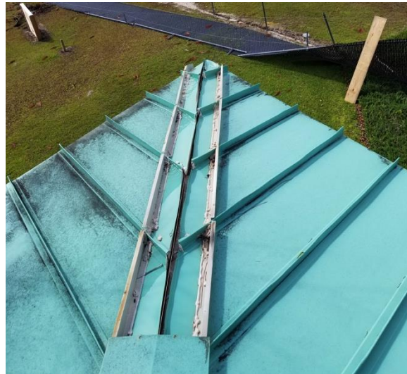
Missing ridge cap
