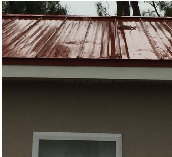
Damage from debris
