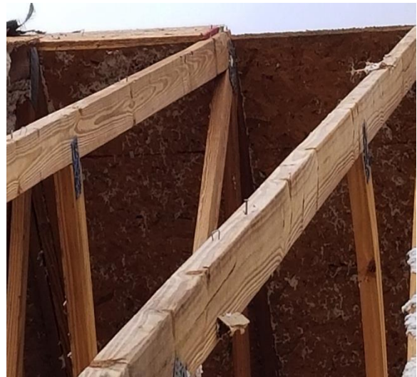
Strange non-code compliant nailing of sheathing
