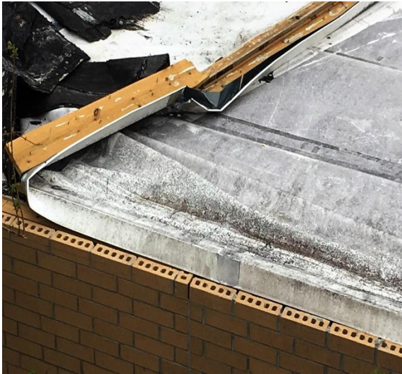
Metal edge dislodged from brick
