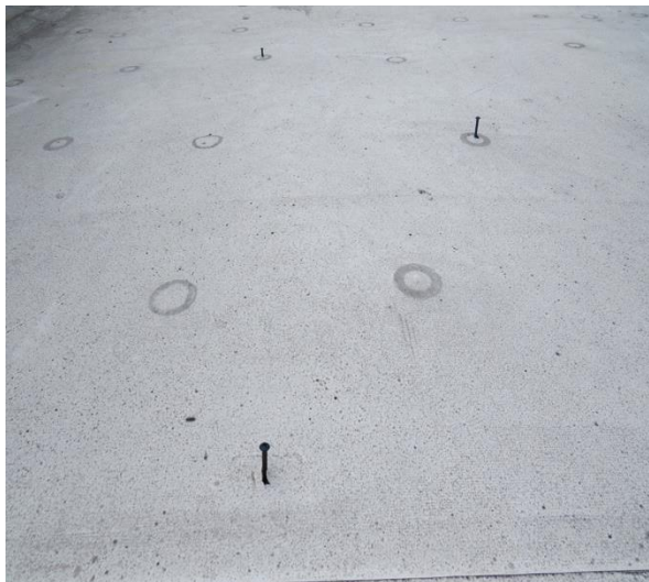
1.2.3 Fasteners that were pulled out due to membrane uplift
