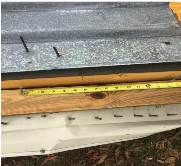
Fasteners that completely missed 2" x 4" nailer that was installed vertically.
