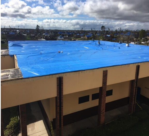
2.2.1 Overview of most damaged area. Membrane and deck dislodged.
