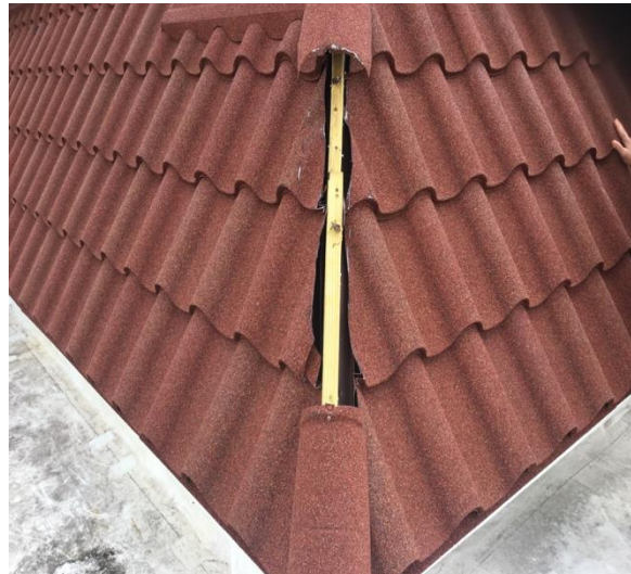
Missing composite Tile
