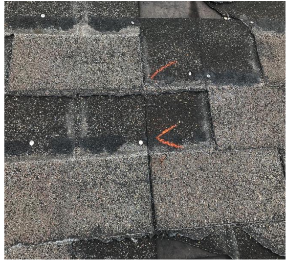
Typical Nailing, nails in sealant strip and missing from one end of shingle
