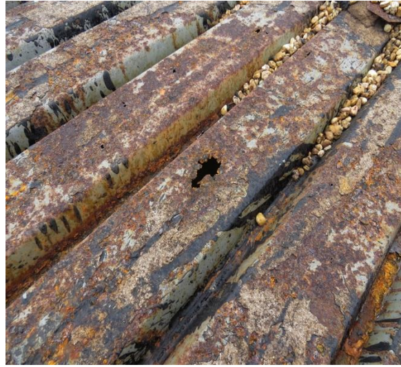
Deck was rusted through indicating earlier leaks
