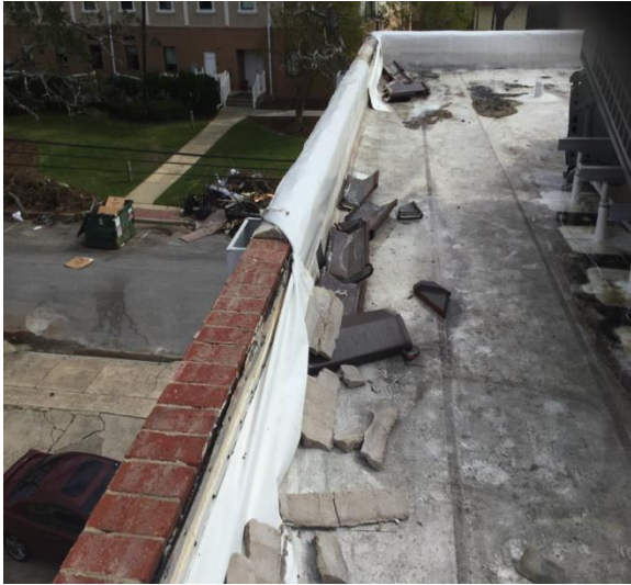
4.2.4 Membrane pulled off parapet and tiles
