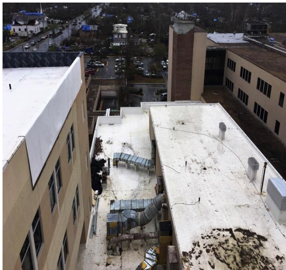
2.1.4 Exterior wall and parapet damaged and a large area of the roof already temporarily recovered. The lower roof was intact, but likely had many punctures from the bricks dislodged from the adjacent building
