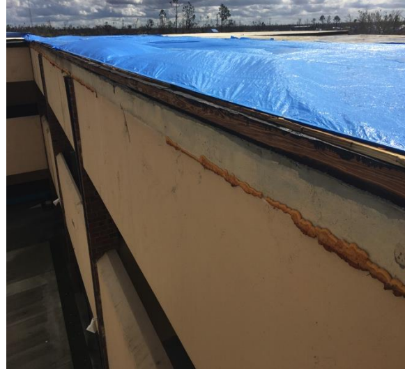
Typical gutter, metal edge and gutter dislodged
