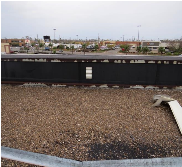
Parapet wall covering missing
