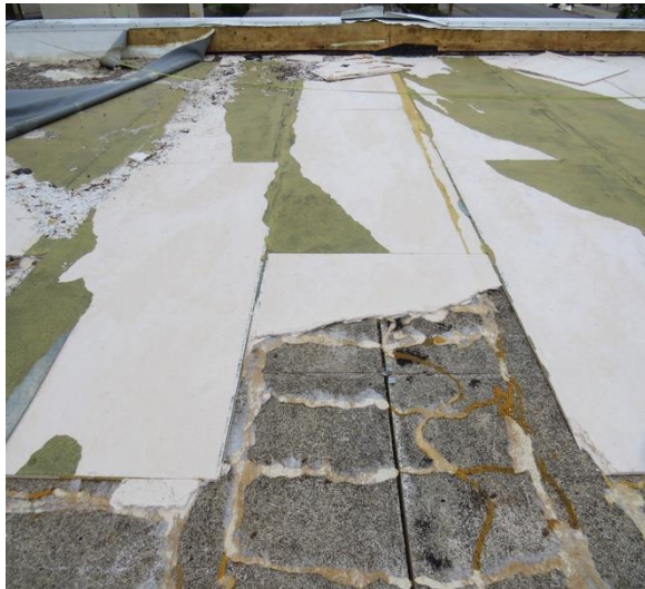
Paper Facer Debonded from Gypsum Board
