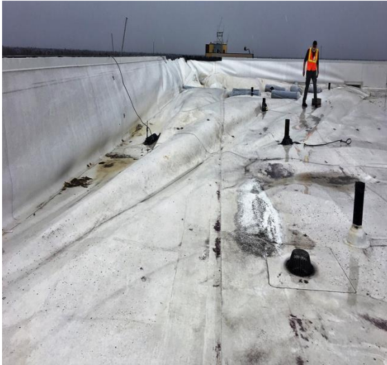
2.1.4 Air is getting into the parapet wall and under the membrane. Significant insulation scuffle
