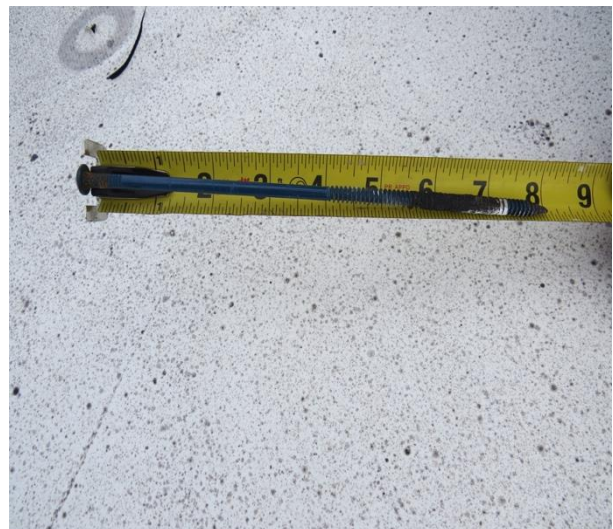
Fastener Corrosion at top and near bottom
