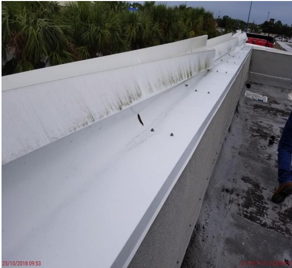
Coping tore over fastener
