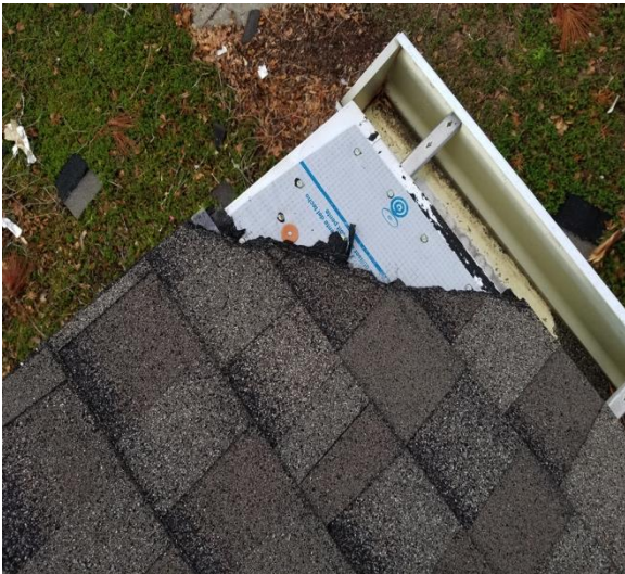
3.1.2 Corner shingles torn
