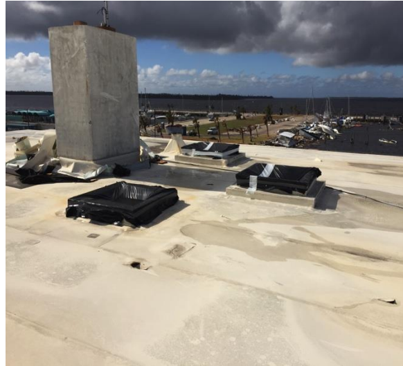
Membrane dislodged from tower
