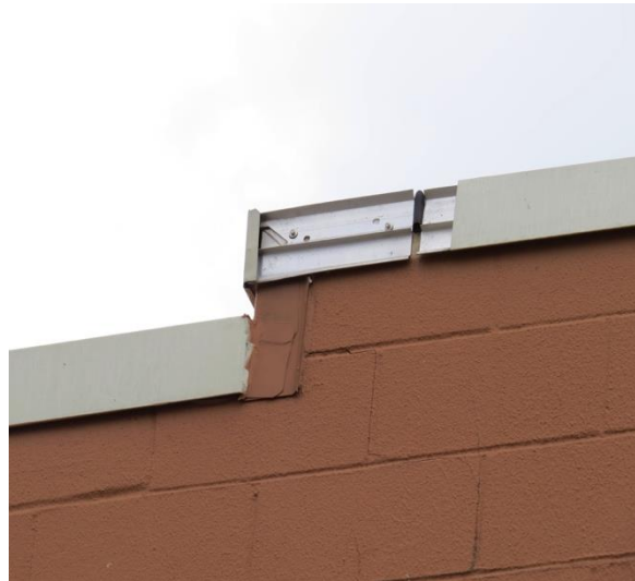
Edge metal missing, not typical
