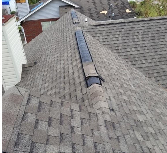
Missing ridge shingles
