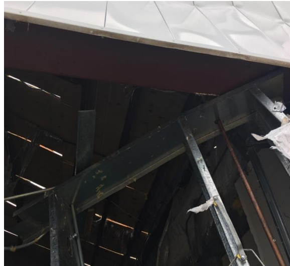
Twisted support beams
