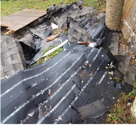
4.1.3 Nails pulled out of sheathing
