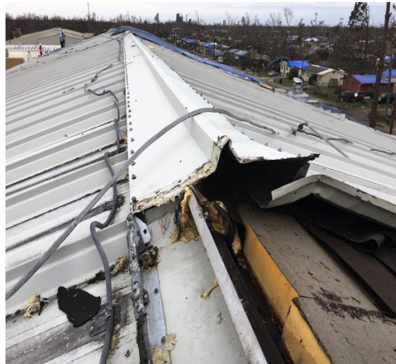
Ridge dislodgement and underlying insulation
