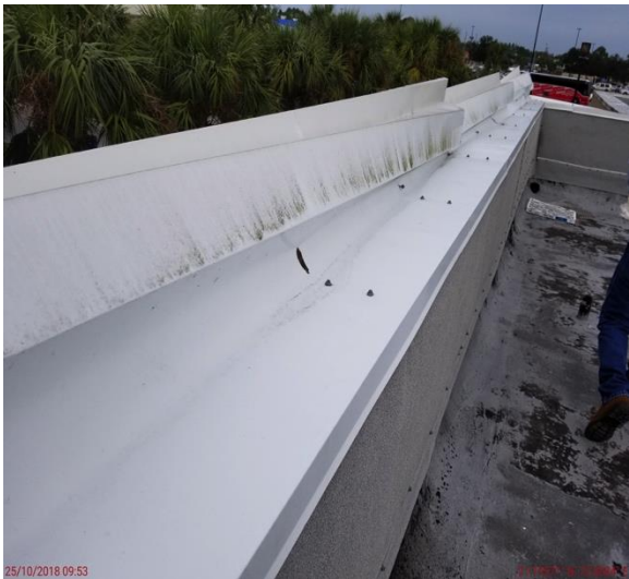
Coping tore over fastener
