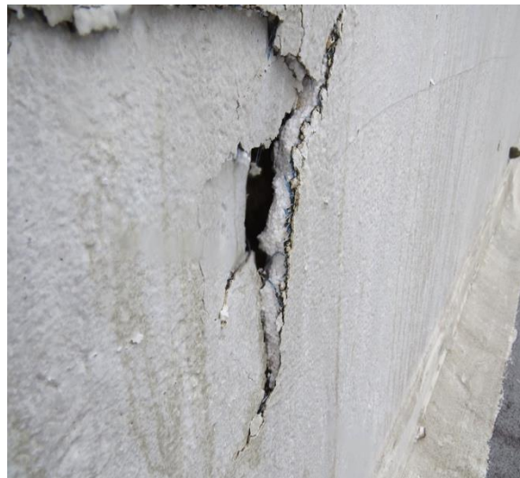
Debris damaged parapet
