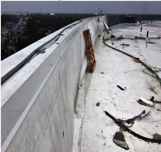
High parapet billowed
