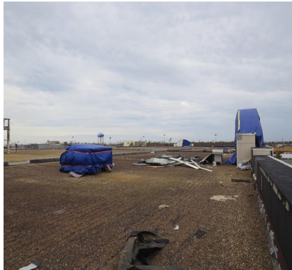
Missing wall covering
