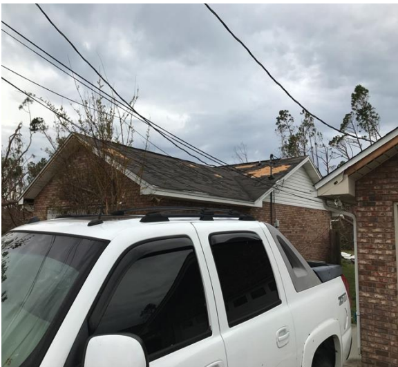
3.1.1 Shingles missing from all sides
