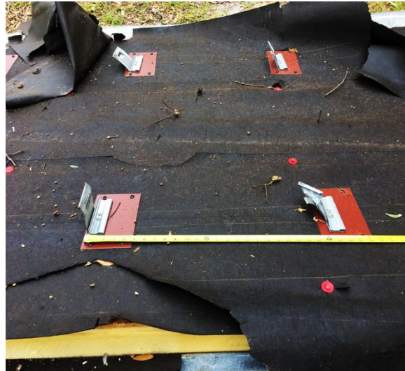
System: Standing seam, 2.75 Iso insulation, #30 felt, Metal deck, all dislodged in some locations
