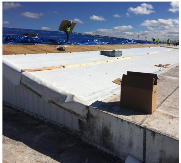
A large section of the standing seam metal roof and the single ply cover was dislodged in this steeper roof area.
