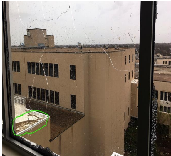
Gravel & debris that accumulated on lower roof
