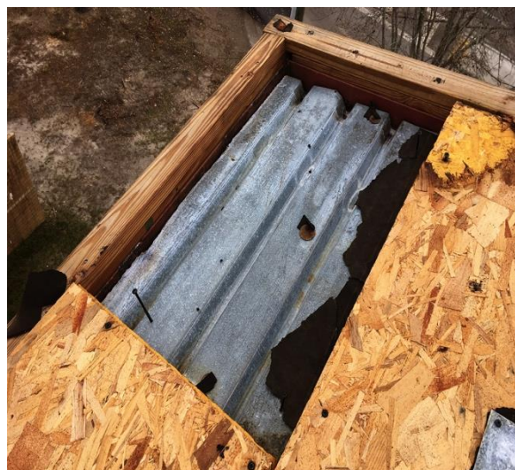
Dislodgement down to deck
