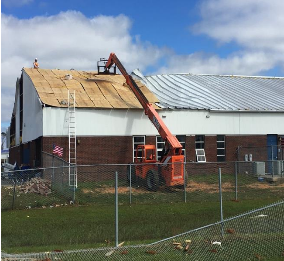
2.2.3 Overview: Missing & bent panels
