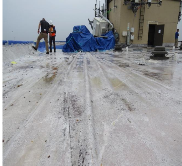
Membrane dislodged from parapet
