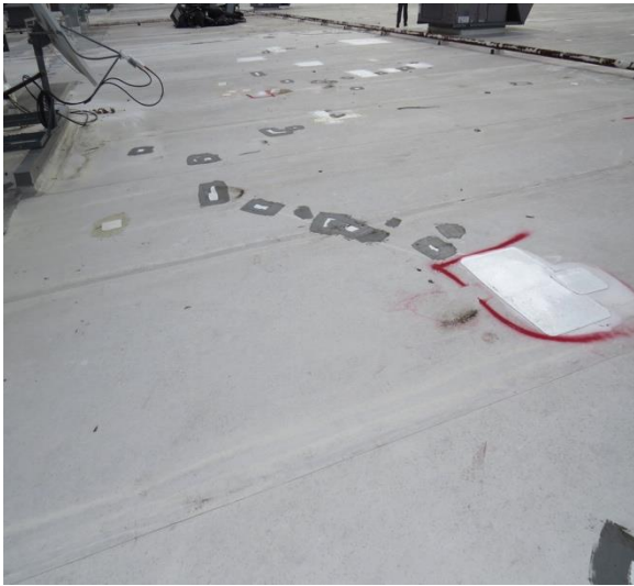
1.1.1 Trail of puncture damage from dislodged
