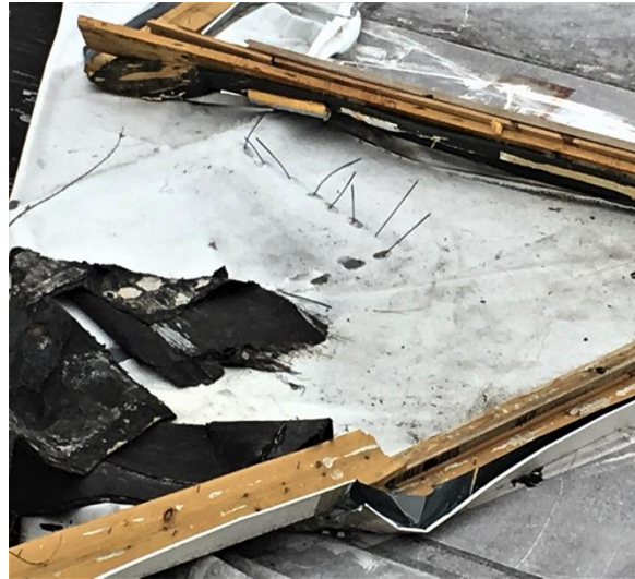
Nailers not adequately fastened to building
