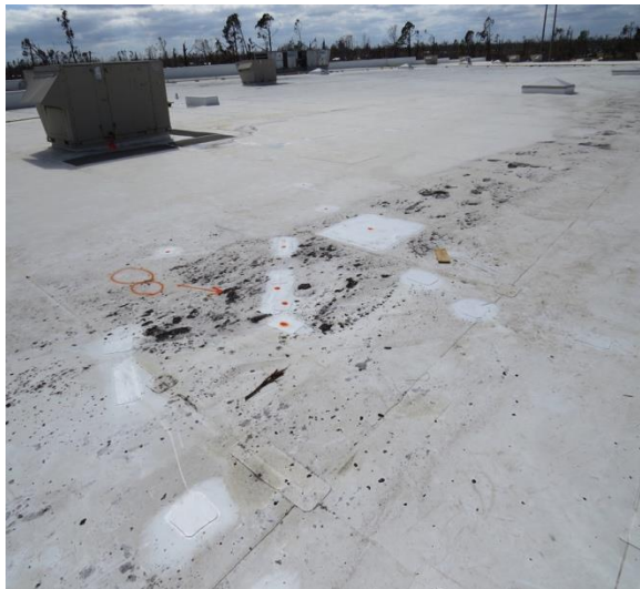
1.2.5 Trail of damage
