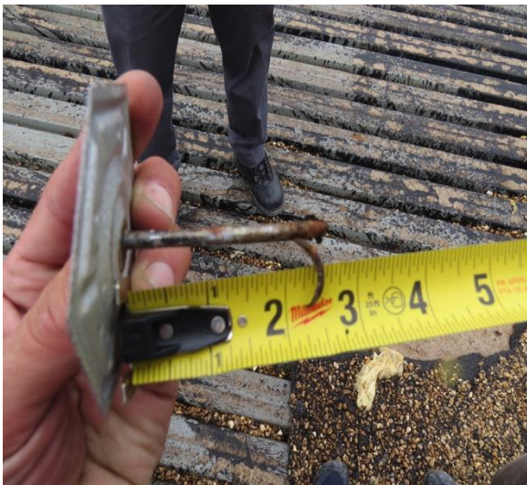
Fastener used to attach Iso to perlite through original gravel surfaced built up roof (BUR)
