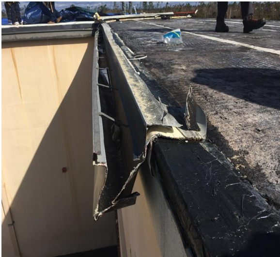
Gutter and metal edge dislodged
