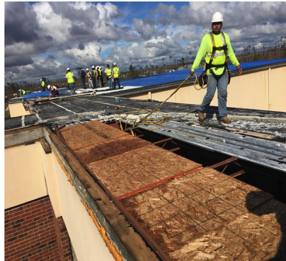
Complete system including membrane lightweight concrete, underlayment board and metal deck dislodged
