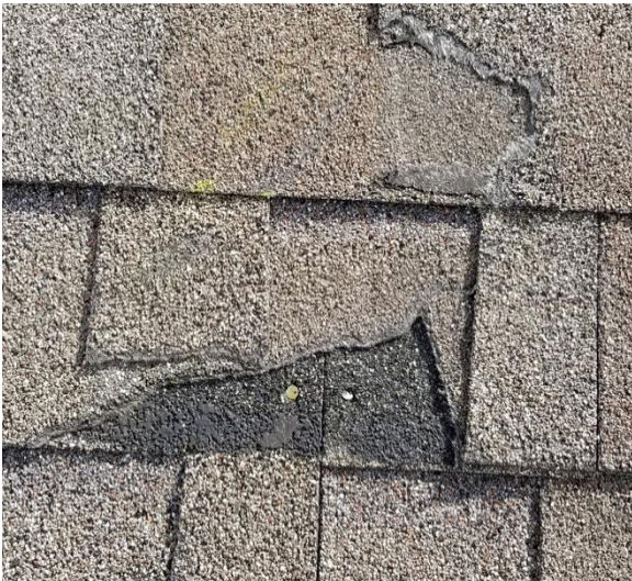
3.2.3 Broken Shingle - nailing
