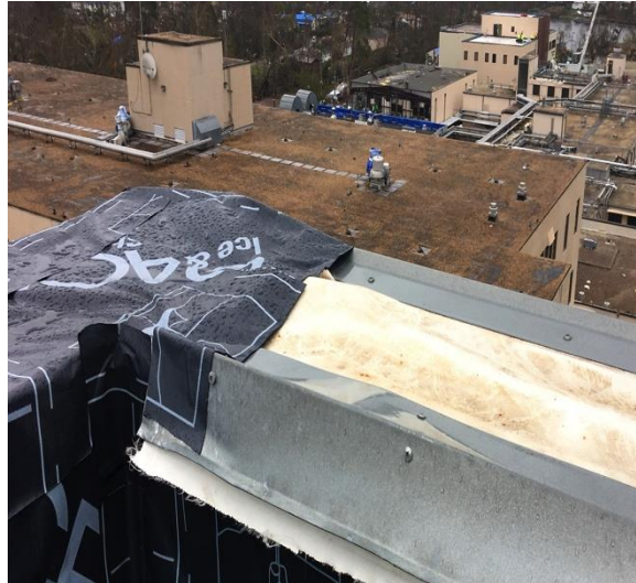
Coping cleats intact, but coping missing
