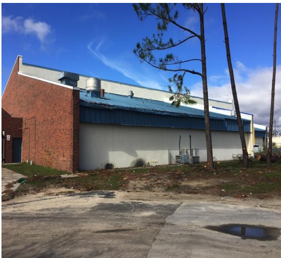
Edge damage; some due to trees and other to uplift
